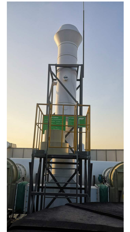
Waste gas treatment facility
